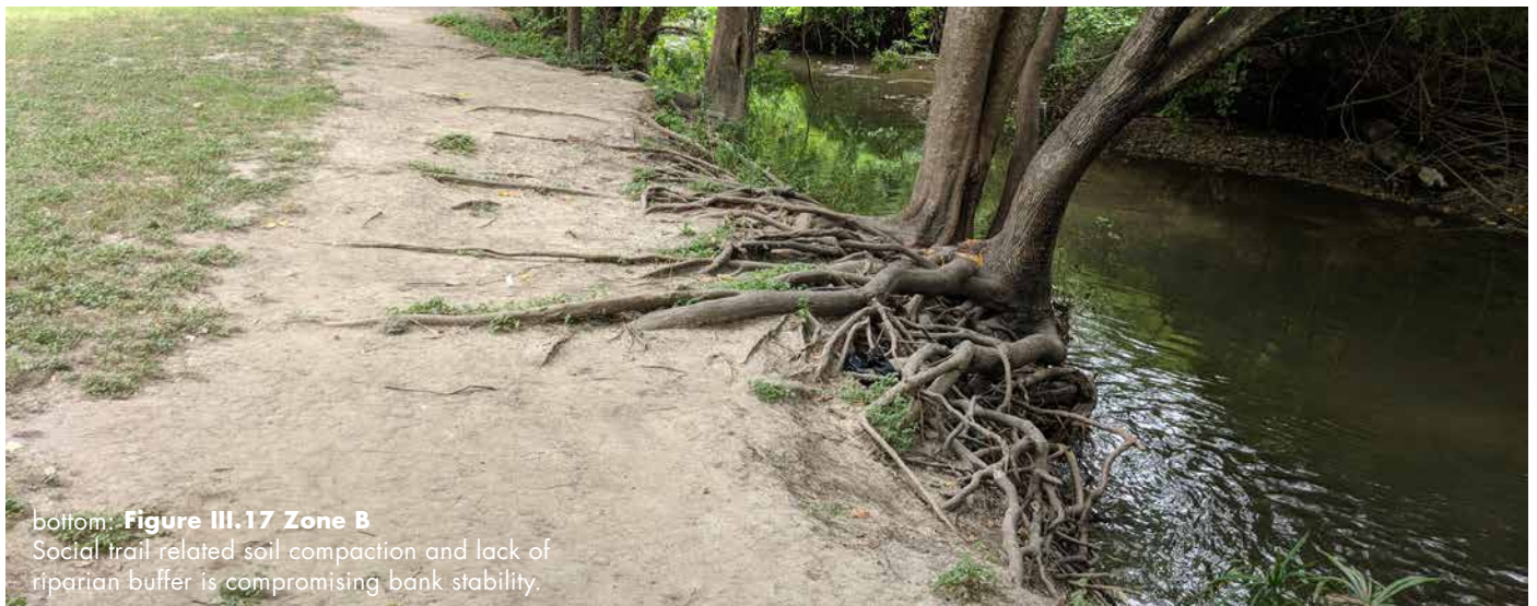
middle: Figure III.16 Zone B Eroded bank lacking root mass
