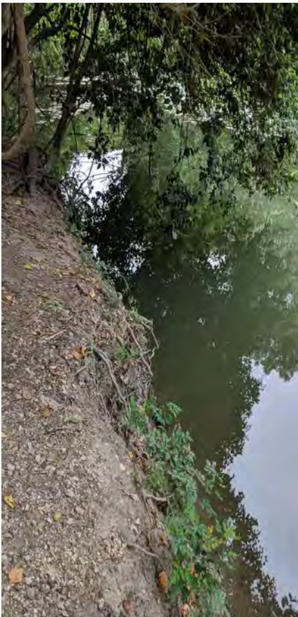
top: Figure III.28 Zone F Riparian vegetation as been removed for access, resulting in accelerated erosion
