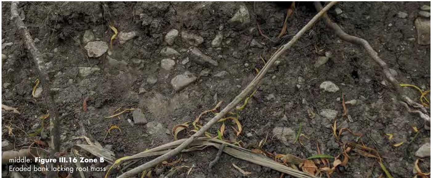
top: Figure III.15 Zone B Compacted and eroding bank. Compacted soil limits root growth, reducing bank stability.
